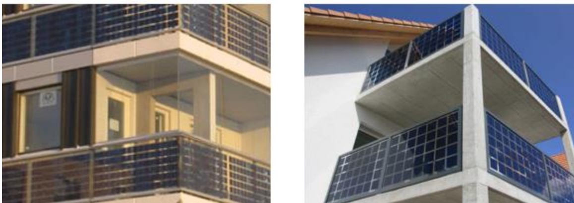
Figure 16. Integrated Photovoltaics applied as an architectural element on the Balcony
