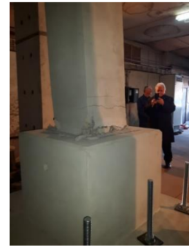
Fig. 3. Heavy damage at PC column (footing safe)
