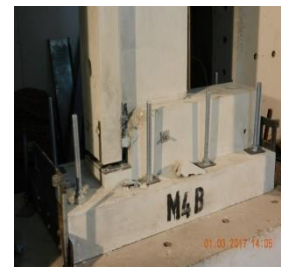
Fig. 18. Failure of improved original connection M4-B
