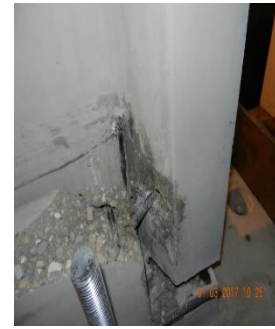
Fig. 15. Final failure state of original connection M4-A
