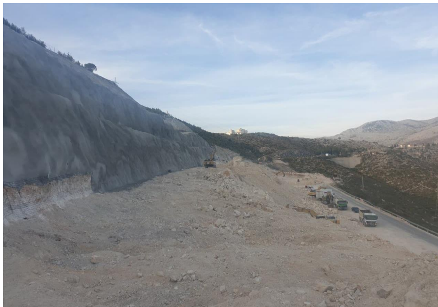
Figure 3. Protection of slopes with shotcrete, anchors and reinforced network on the expressway Prilep-Gradsko
